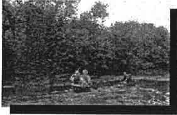
Figure 44. One of many abandoned rail bridge supports along the lush river banks.
